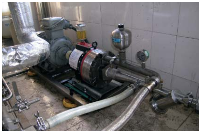
Pharmaceutical processing facility.
